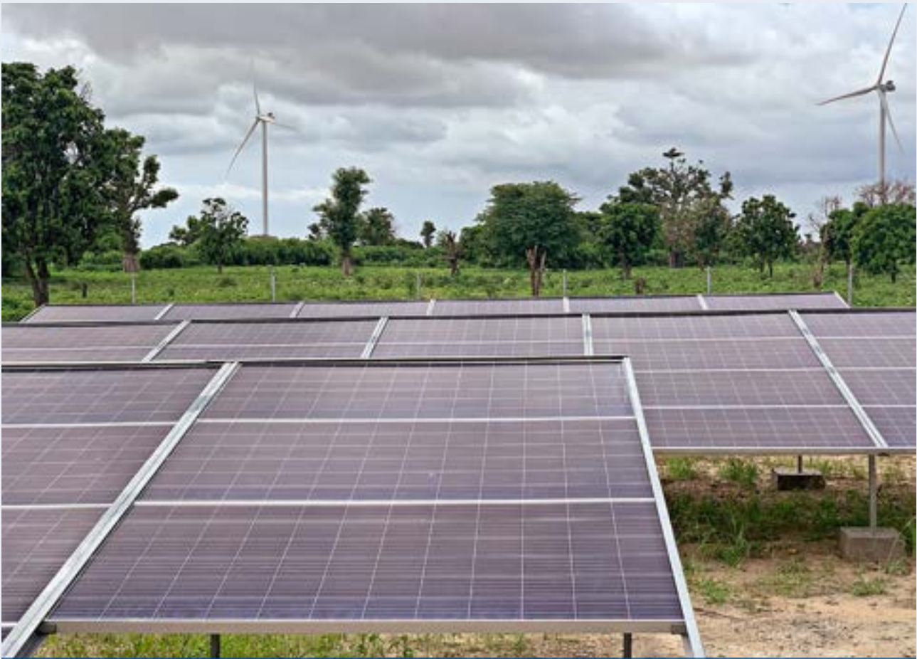
Solar power for the water pump in the eight villages near Tobene Power
