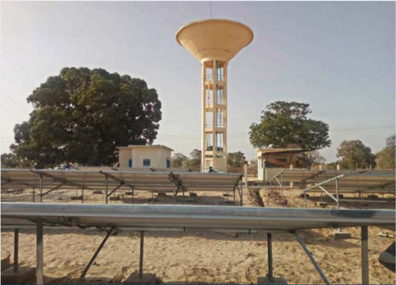
Solar power for the water pump in the eight villages near Tobene Power
